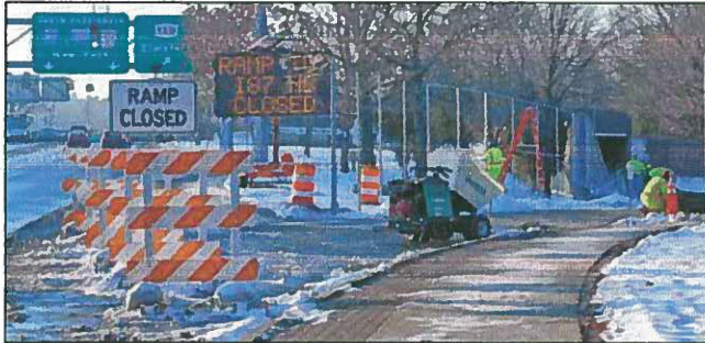
Closure of ramp to bridge has created much frustration for local motorists.
